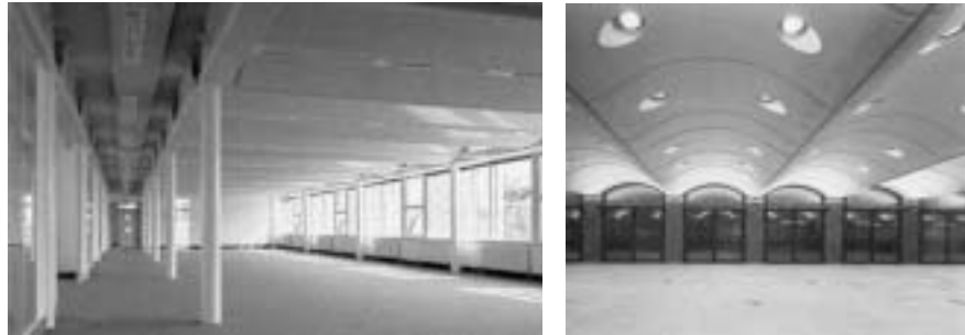
Figure 7.77 The soffit to the sinusoidal concrete slabs are left exposed in the interiors of both The Environmental Building of BRE in Watford, UK ( left ) and in the Inland Revenue Headquarters in Nottingham, UK ( right ). The upper side of the sinusoidal concrete slabs provide horizontal air paths, and the sinusoidal design provides large areas of thermal mass.
