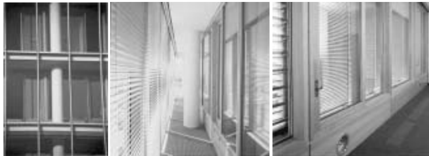
Figure 7.20 The outer skin of the double façade of the administration building of Deutsche Messe AG in Hanover ( left ) protects the inner wood and glass façade ( middle ) against the weather. Sliding French windows provide inlets for the natural ventilation ( right ).
