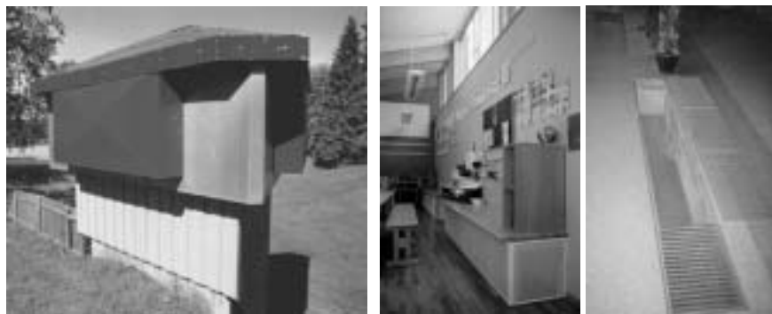
Figure 6.9 The inlet tower ( left ) and the low-velocity diffusers in the classrooms ( middle ) and the inlets in the common rooms integrated in the floor ( right ).
