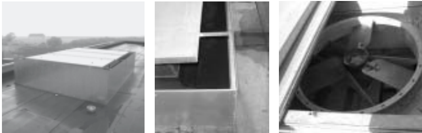
Figure 5.15 One extract cowl is located over each of the two stairwells ( left ). The cowls are made with a slit running around the top perimeter of the cube to utilise wind suction regardless of wind direction ( middle ). Two axial fans are located in each of the two cowls ( right ).
