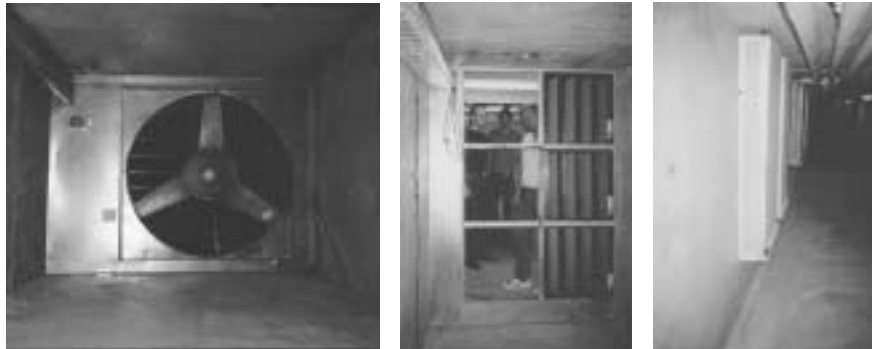
Figure 6.11 The panel of filters (six in all, the three cassettes to the left are removed in this picture) in the end of the embedded supply duct ( left ), the sound attenuators in the distribution chamber ( middle ), and the extract fan in the exhaust tower ( right ).
