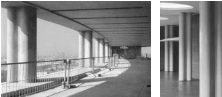
Figure 4.7 Picture taken under construction of the high-rise showing the structure ( left ). (Concrete/steel columns carry a post-stressed RC edge beam between which prefabricated floor elements span). The picture shows how daylight that enters from the side modulates the shape of the columns in the conference room of the baguettini ( right ).
