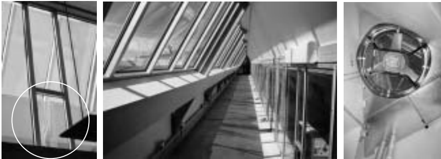
Figure 6.10 Motorised glass-hatches (encircled left ) lead exhaust air from the classrooms and into the extract chamber ( middle ). The extract fan is located high up in the exhaust tower ( right ).
